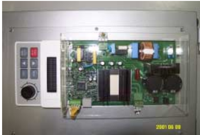
(a) Control board
